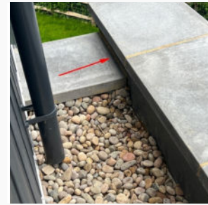
Mortsr cracking on tiles 25/05/2022 11:13 (BST)
