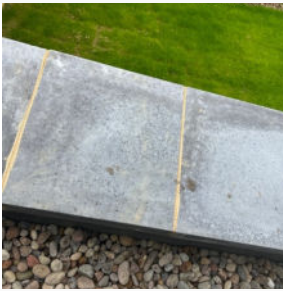
Excess mortsr on tiles 25/05/2022 11:13 (BST)
